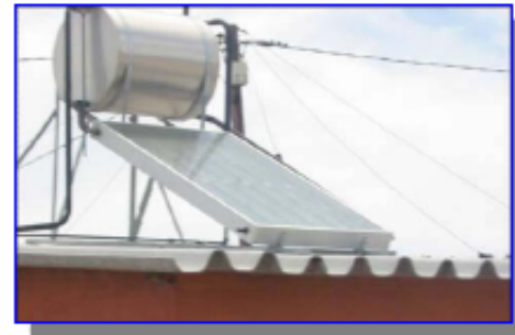
Solar water heaters
